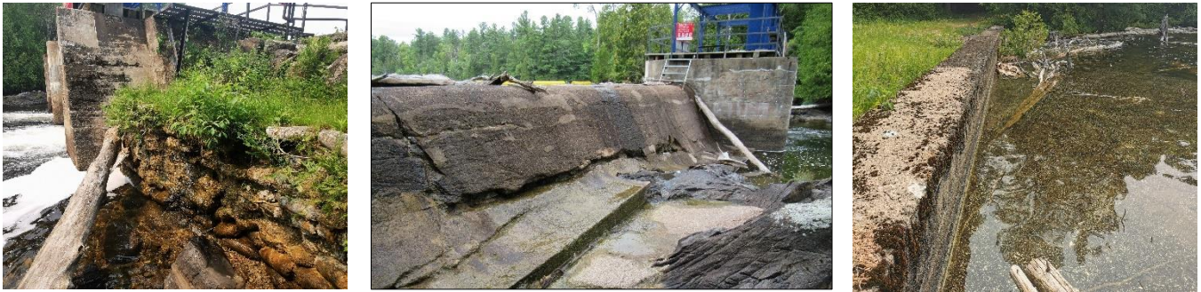
Photos: South abutment wall (left), overflow weir (middle), and saddle dam (right).
