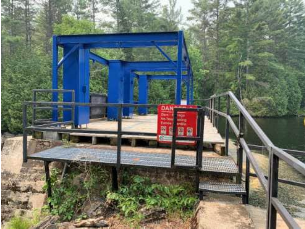
Photo 1: Existing conditions of the Kashwakamak Lake Dam structure to be replaced, facing north.
