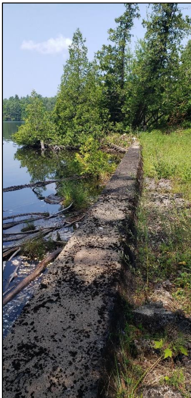
Image 12. View of disturbance caused by construction activities in the northern portion of the study area, facing southeast. (PR23-021D041)
