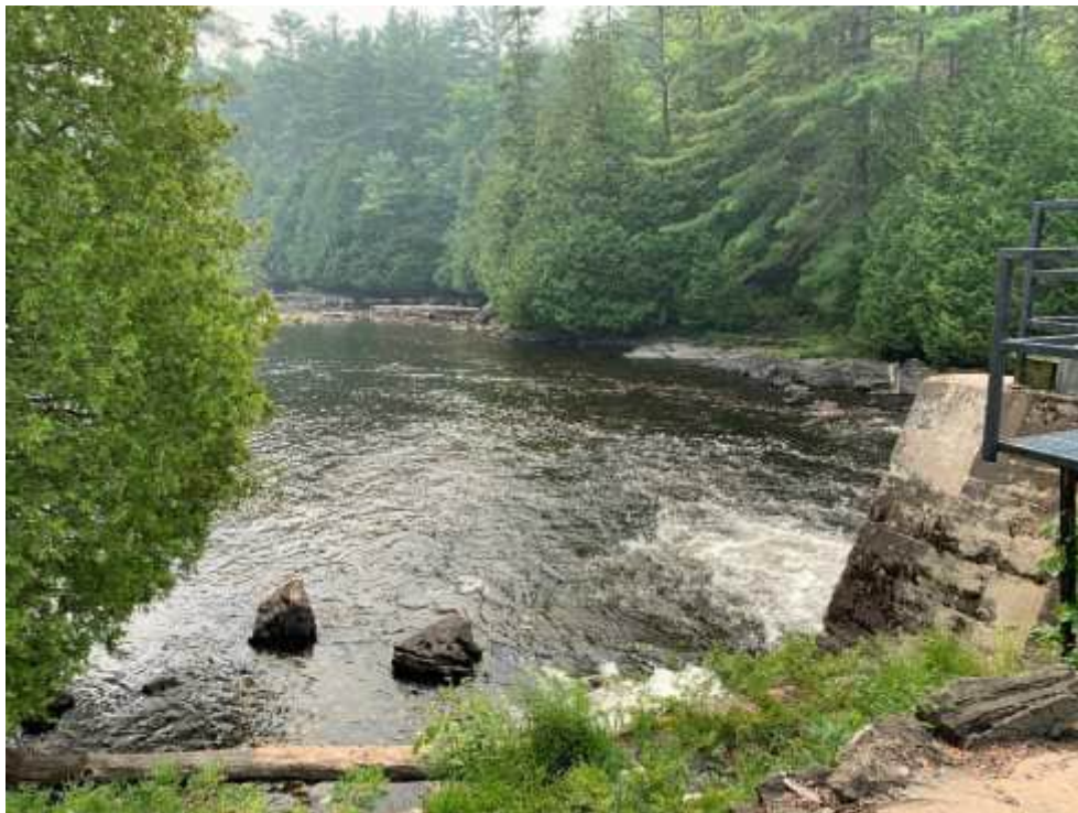
Photo 2: Existing conditions of Kashwakamak Lake, downstream of the dam structure. Facing east.
