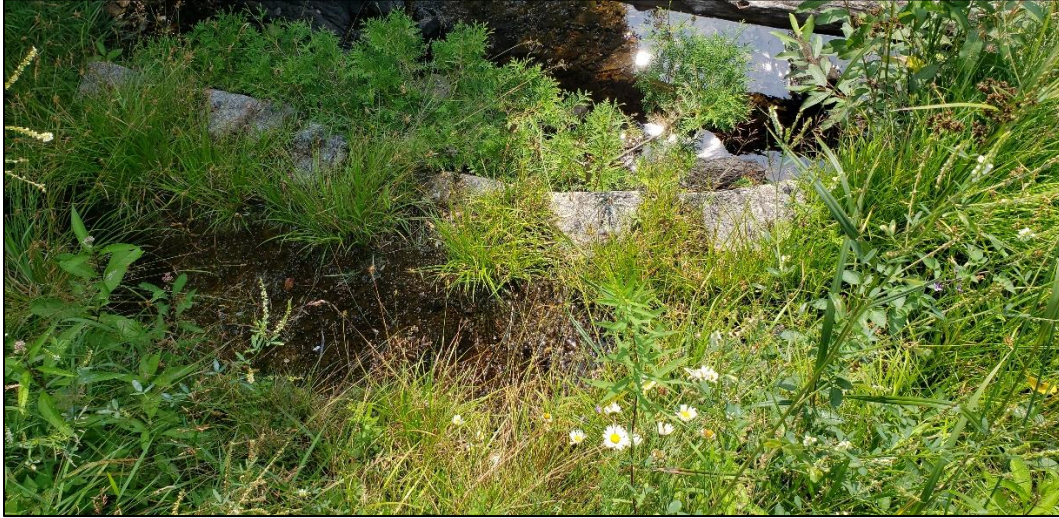
Image 7. View from above of the retaining wall at the north end of the control dam, facing east. (PR23-021D013)
