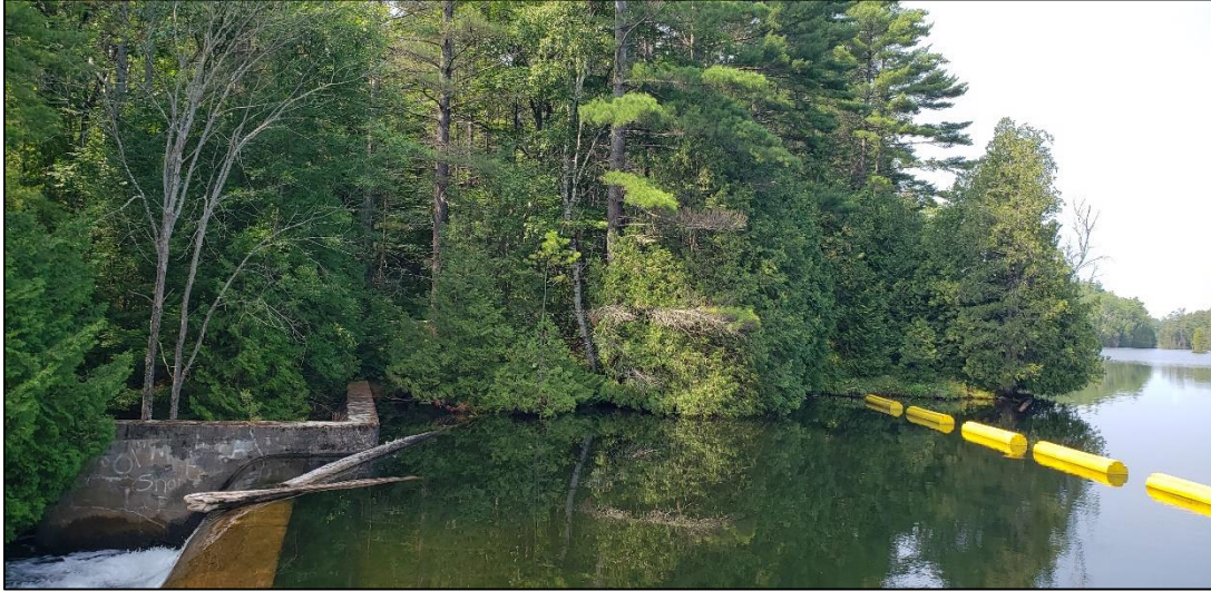
Image 11. View of the southern shoreline at the control dam, facing southwest. (PR23-021D007)
