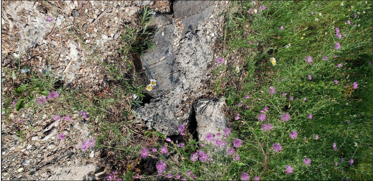
Image 9. View of a secondary patch of concrete fill at the northern end of the control dam, facing east. (PR23-021D014)
