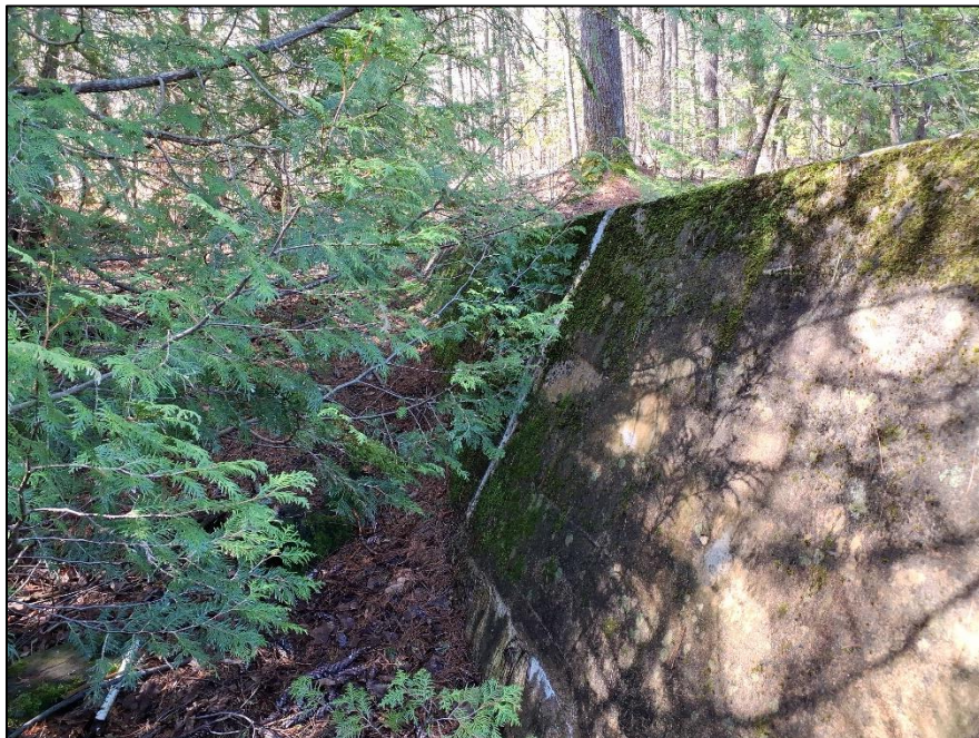
Image 29. View of the south side of the control dam, facing southwest. (PR23-021D086)
