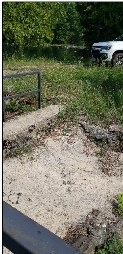
Image 8. View of the main patch of concrete filling in the approach to the northern end of the control dam, facing northeast. (PR23-021D012)
