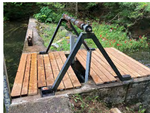
Mississagagon Lake Dam Safety Controls
