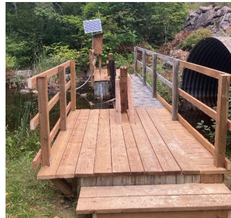
Pine Lake Dam Safety Controls
