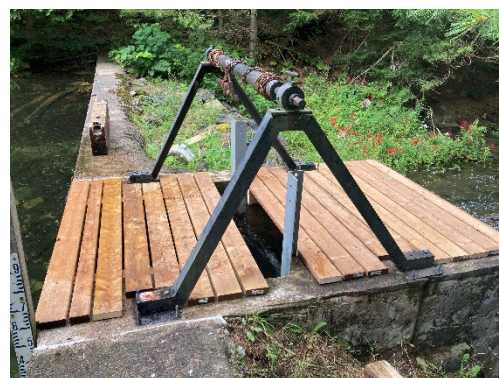
Mississagagon Lake Dam Safety Controls
