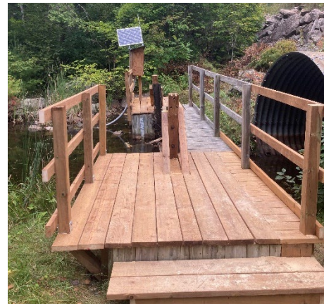
Pine Lake Dam Safety Controls
