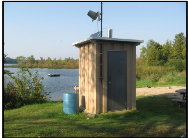
Bennett Dam Gauge
