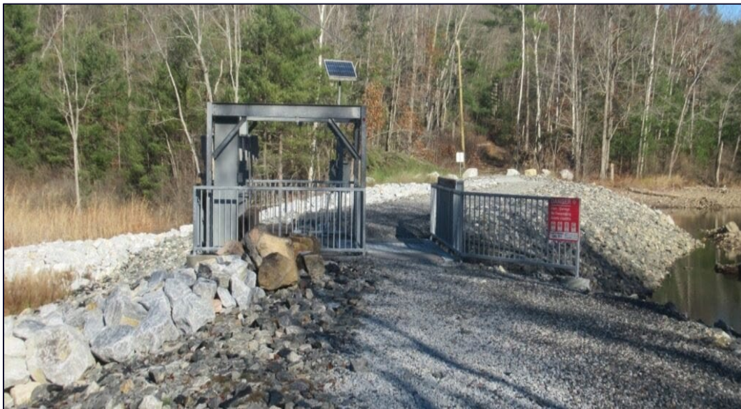
Recently rehabilitated Shabomeka Lake Dam deck and embankment with new safety railing
