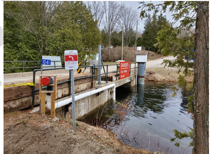
Dry hydrant at Palmerston Lake Dam
