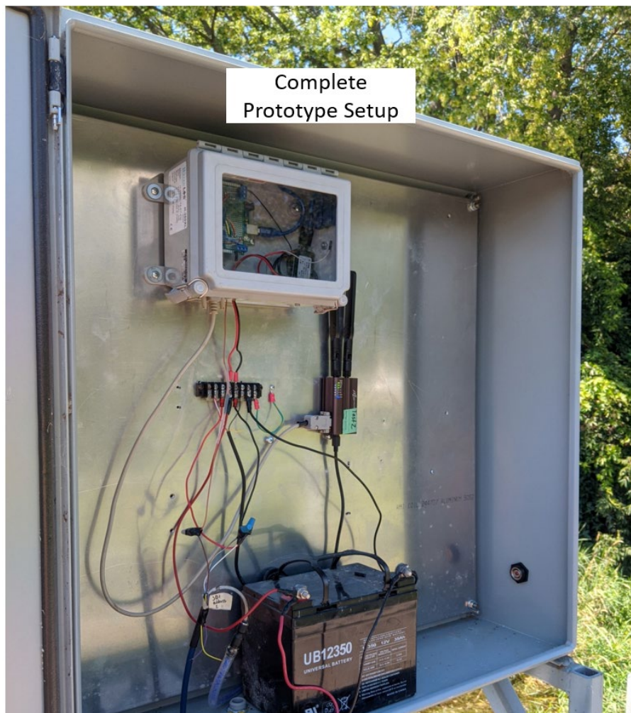
Figure 2 - Datalogger (top) with cellular modem (middle) and battery power (bottom) installed at Carleton Place Dam.
